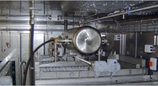
Snow Removal System (SRS)
